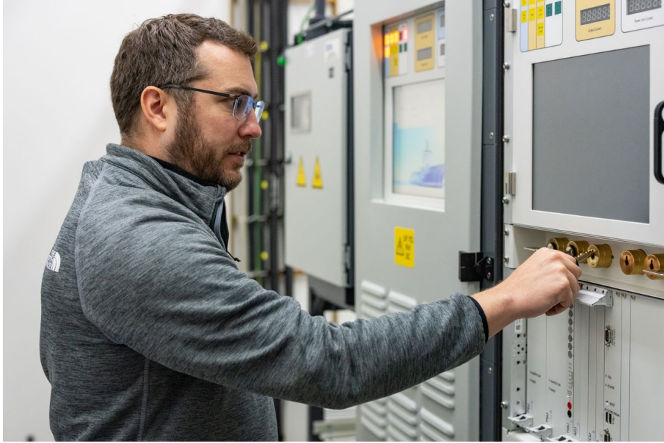
Pictured: An Alaska Communications technician inspects new power feed equipment (PFE) and one of the company's cable landing stations.
